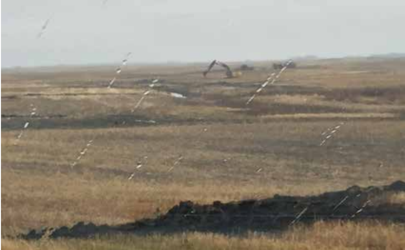
Figure 8. An example of intensive ditching construction targeting multiple wetland basins in a cultivated field.
